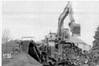
Construction crews grind up concrete on the site of the old Central Middle School on Tuesday morning as the demolition continues. The Sheridan Press/John Carroll
